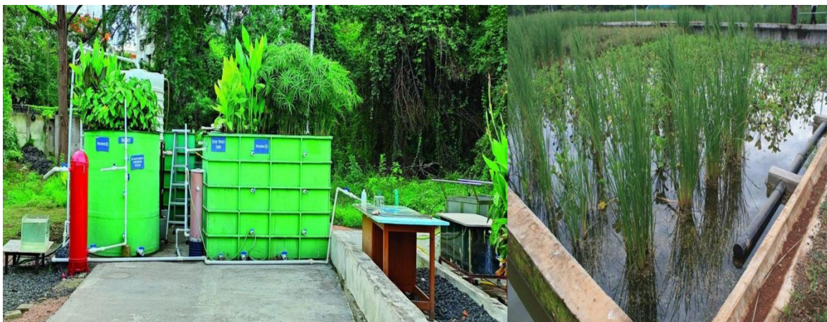
Figure 3 Reed Bed-Based Decentralized Wastewater Treatment Ujjain (Ravindra Nagar) | Nature-based treatment system. (Source: Google)
